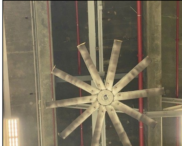
Spalling on concrete hangar roof at Air Station Cape Cod, MA
