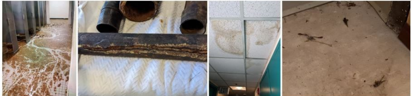
Sewage overflow in training barracks restroom
